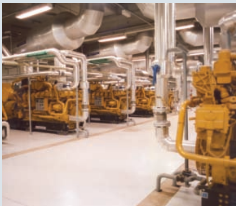
© Unibanco | Usina Bandeirantes thermoelectric plant in São Paulo, Brazil (production facilities) produces clean energy from landfill gas and delivers a substantial amount of carbon credits. The plant is the largest of its kind in the world and was financed by Unibanco.
