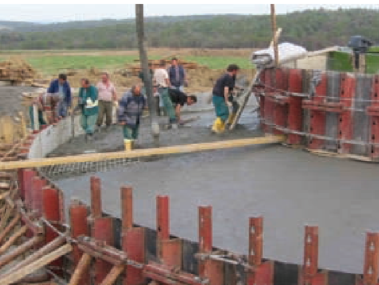
© Martin Dasek, IFC | Workers building the base of a 2-MW wind turbine in Northern Bohemia, a project financed by Česká Sporitelna, A.S. (member of the Erste Group) (see story, p. 18).
